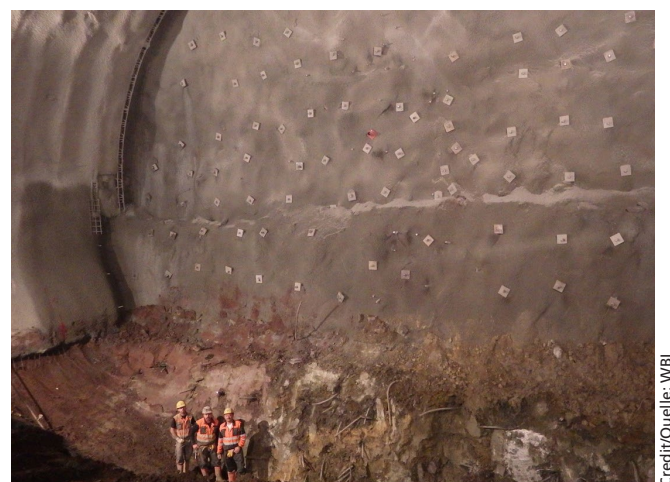
10 Heading central station south, excavation of invert area Anfahrbereich Hbf. Süd, Sohlaushub Credit/Quelle: WBI
